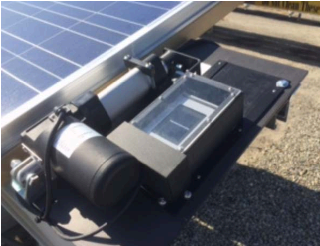
Figure 5: MaxSun Soiling Station
